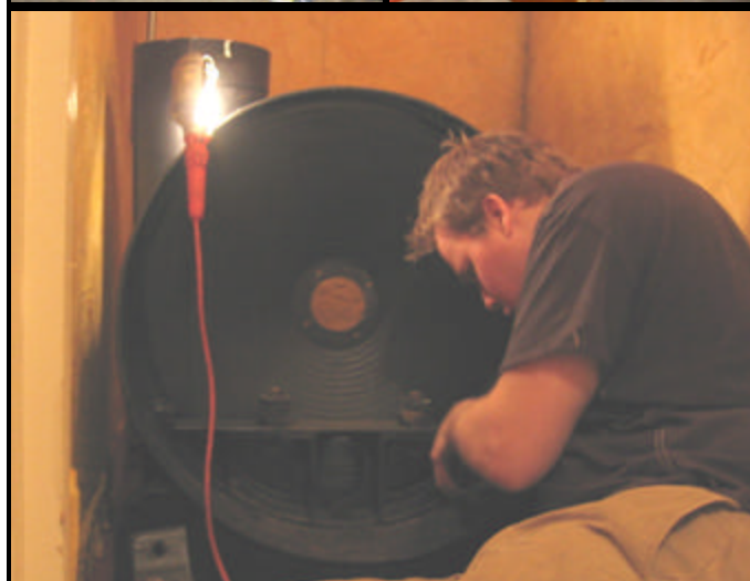
Top: Ed Rickert gathers the tools. Middle: Motor and Blower. Bottom, Dean Rosko works in the confines of the blower room.
